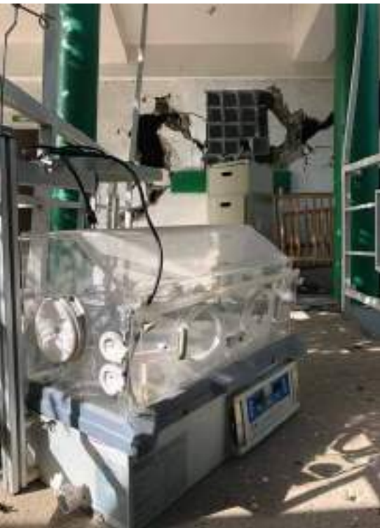
▲ The medical facilities can be easily recognized in Haiti by their green and white color. Many were severely destroyed in the earthquake.
