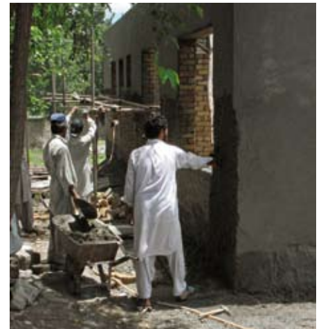
Pakistan: Works on the shell of a health centre in Azad Jammu and Kashmir
