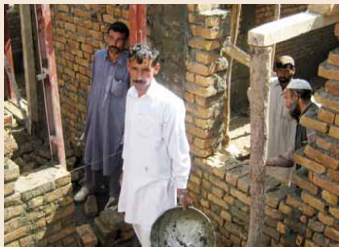
If possible, local workers are employed to reconstruct and rehabilitate health facilities and other social infrastructure projects.
